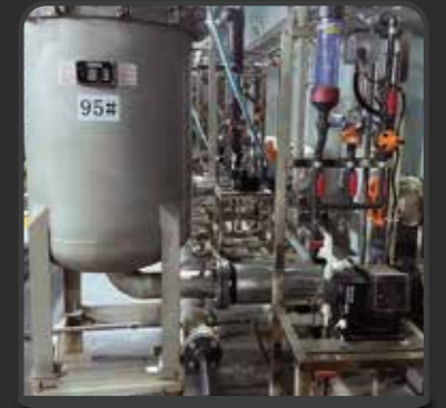
Industrial cooling system scale inhibitor addition
